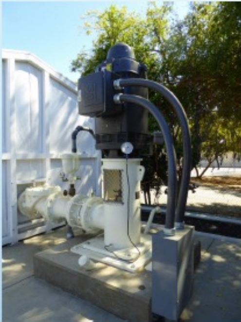
Groundwater Extraction Well
