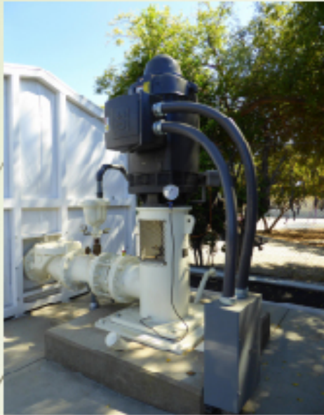
Groundwater Extraction Well
